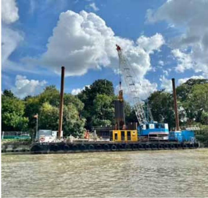
One of our members took this picture of the work taking place at the Thames towpath breach between Kew and Richmond
